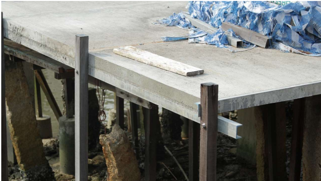
Figure 1. A semi-composite concrete and steel floor, built in place of a burned-down stilt house and subject to work stoppage. Photograph by Daniel Keith Elkin.
