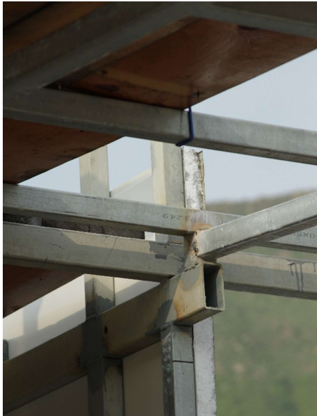
Figure 2. Connections in a newly-rebuilt stilt house. The contractor's use of galvanized steel tube sections led to a work stoppage approximately sixty days long. Photograph by Daniel Keith Elkin.
